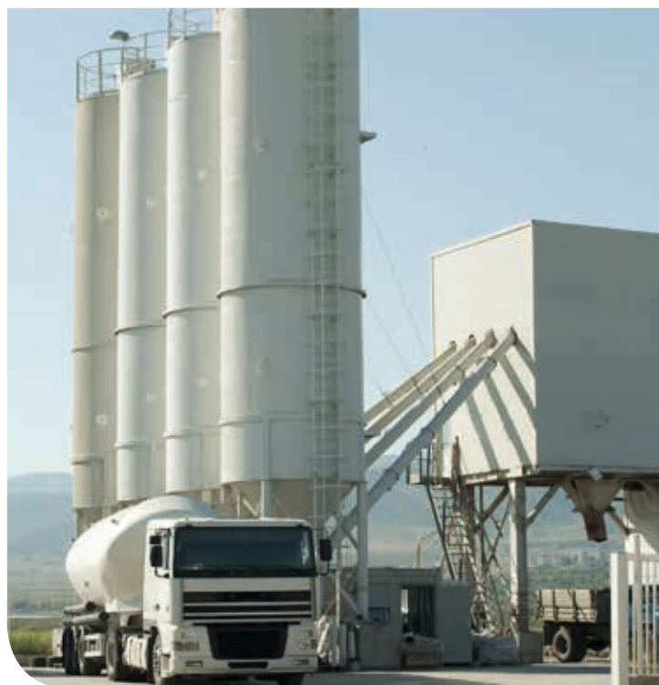
Delivery of plastic granules & filling of silos using pneumatic conveyors
