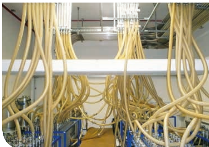
Distribution station (hose station), forwarding of raw materials for granule drying
